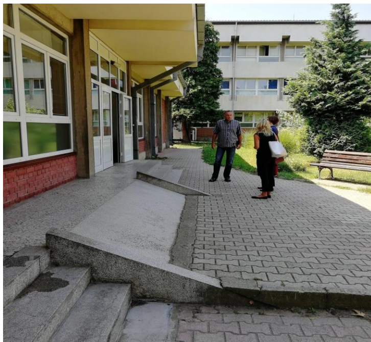
Image 14 – Children’s clinic in Trstenik: an example of a useless and unsafe ramp
