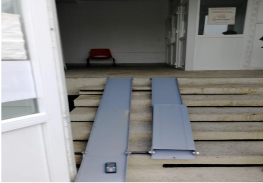
Image 10 – the center for social work in Blace: the mountable ramp which is not in compliance with the standards and the office for reception of the parties with serious difficulties in movement
