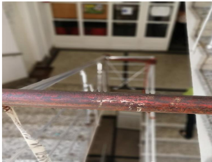
Image 20 – The PDI fund in Prokuplje is located in the attic of the facility shared with a few more owners; the adaptation of the offices has recently been done and the replacement of handrails at the staircase is obviously inadequate so it was necessary to additionally install one part of scaffold for fixing and the stability of the handrail but the premises of the Fund are still inaccessible to the citizens with difficulties in movement because there is no elevator and movable platform;
