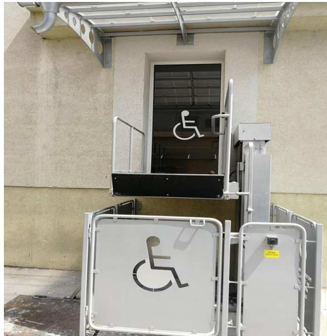
Image 19 – The affiliate of the PDI fund in Kraljevo: the lifting platform at the lateral part of the building without visible labels and guideposts which could attract the user's attention. Additionally, the platform is designed in such a manner that its independent use is impossible
