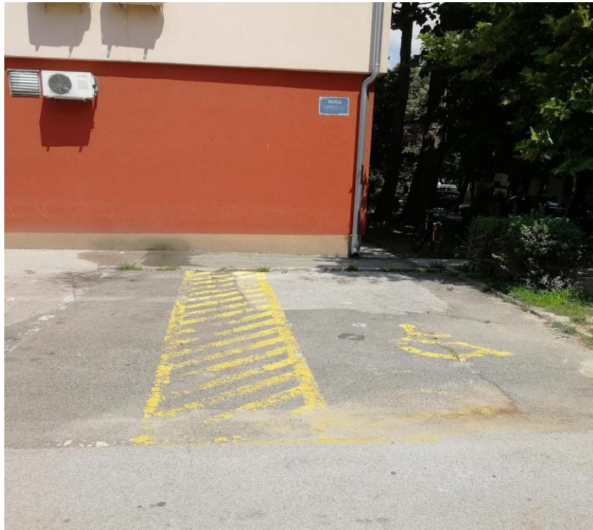
Image 7 – The Health center Apatin –the parking lot for persons with disabilities without vertical signalization placed at the greatest distance from the entrance to the facility instead of being at the shortest distance
